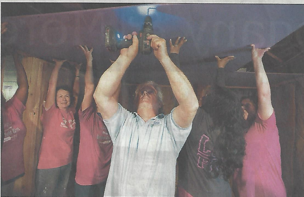
CHRIS PEDOTA/STAFF PHOTOGRAPHER Chris Warburton of Habitat for Humanity showing United Water workers how to put up drywall.
