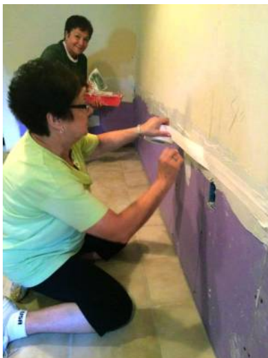
PHOTO COURTESY OF HABITAT FOR HUMANITY OF BERGEN COUNTY Volunteers at Hudson City Savings Bank recently volunteered to help restore two Hackensack job sites damaged by Superstorm Sandy.
